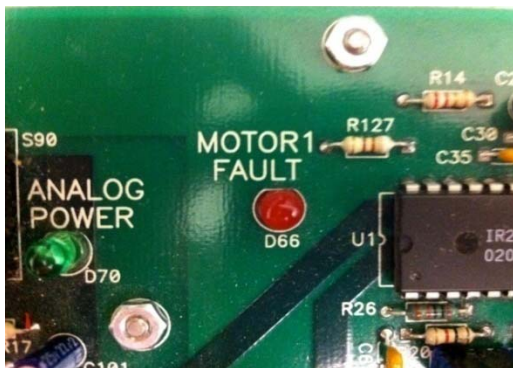
Figure 7(a): Motor-1 Fault Indicator
