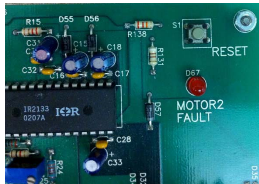
Figure 7(b): Motor -2 Fault and Reset Switch
